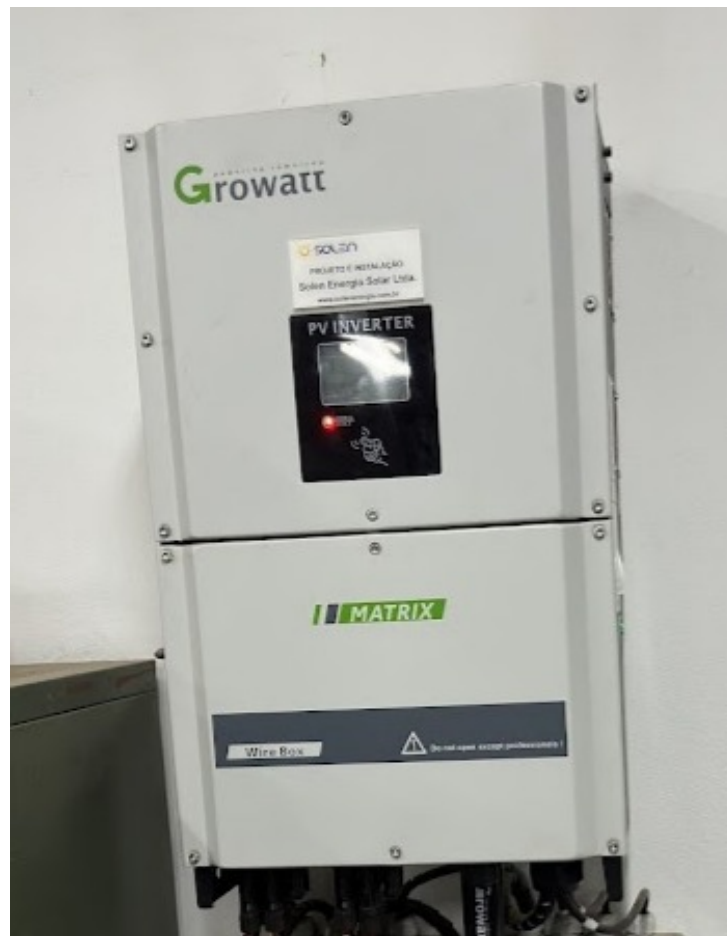
Figura 19 – Inversor – IFMG Campus Itabirito
