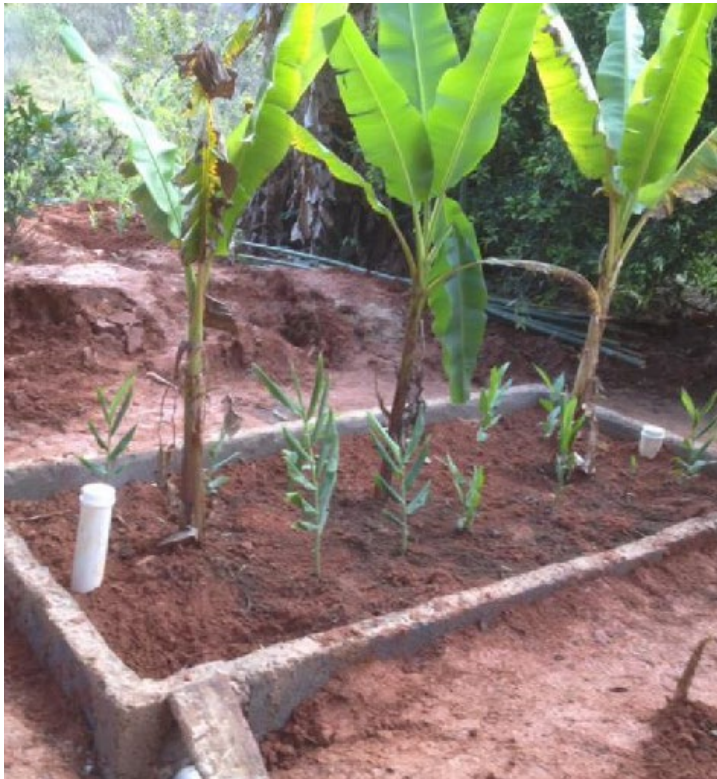
Evapotranspiration Tank (TEvap) or ecological septic tank Source: courtesy photo
